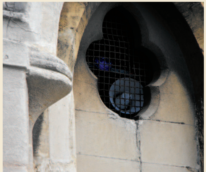
Alarm sounder and blue strobe light installed in a church tower
