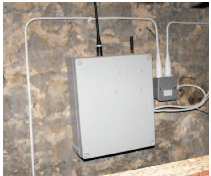
Roof security system panel installed in a church tower
